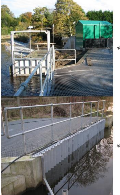
Figure 1- Images provided by Whitby Esk Energy. The Intake System with a View of the Fish Pass (a). The Inlet Screens at the Mouth of the Intake System (b).
